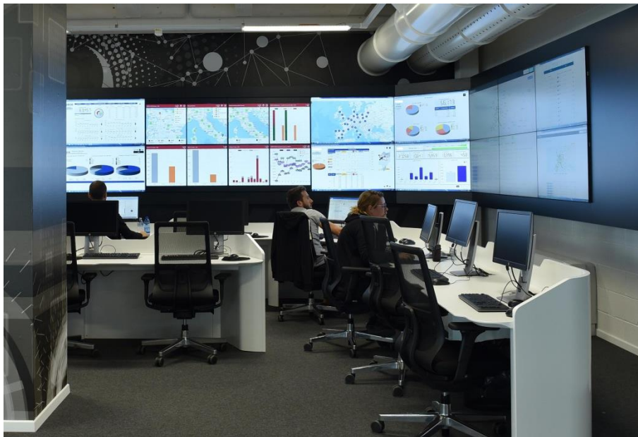
The Control Room
