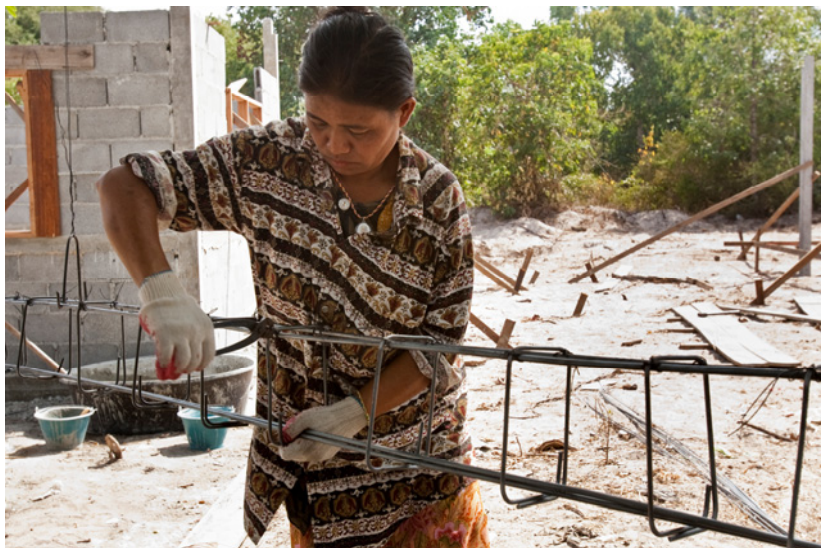
A woman, widowed by the 2004 tsunami, receives help from volunteers to rebuild her home on the island of Koh Kho Khao, Thailand. Thai Rotarians coordinated a national relief effort, and Rotary established a fund to support long-term recovery efforts in India, Indonesia, Sri Lanka, and Thailand.
